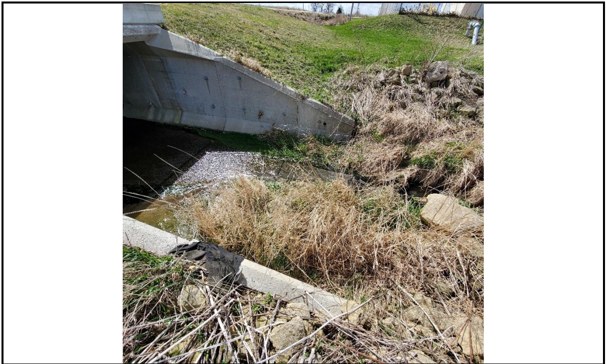
Photo 26: View looking at concrete culvert on south end of Wetland Area 6 under 21 st Street.
